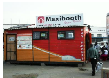
Public phone booth in Zimbabwe, powered with solar panels (left), battery banks for powering billing equipment and phones (right),
